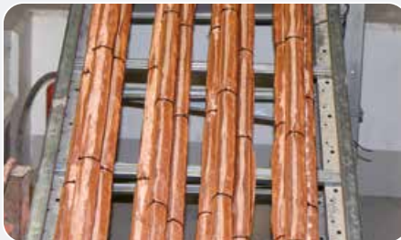
Power cables, data and supply lines
