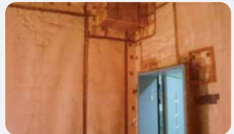
Shielded Rooms and Shielded Chambers
